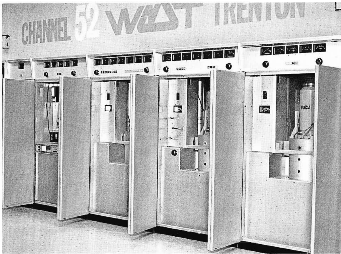
TTU-60B, 60 kW UHF Transmitter used for WNJT-TV test of unattended operation.
